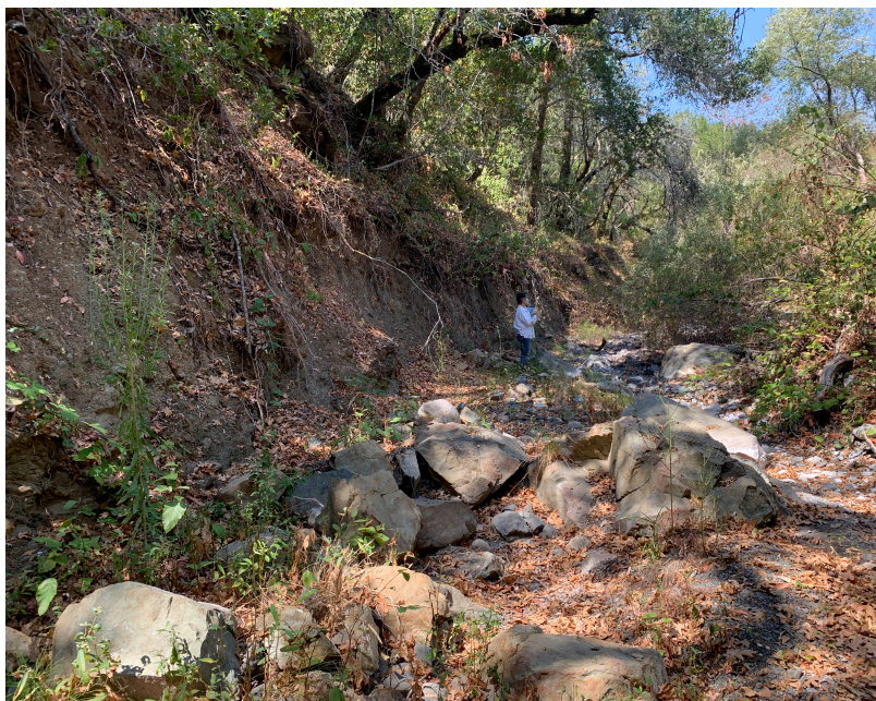
Photo 4 – Over-steepened southern bank and channel bedload (looking west)
