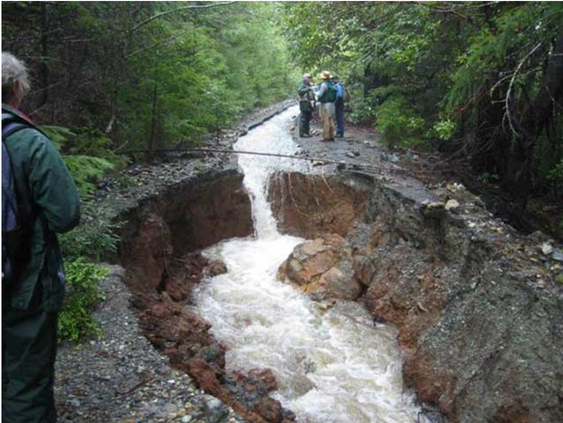
Stream Diversion due to plugged culvert on abandoned road. Source: U.S.D.A Forest Service.
