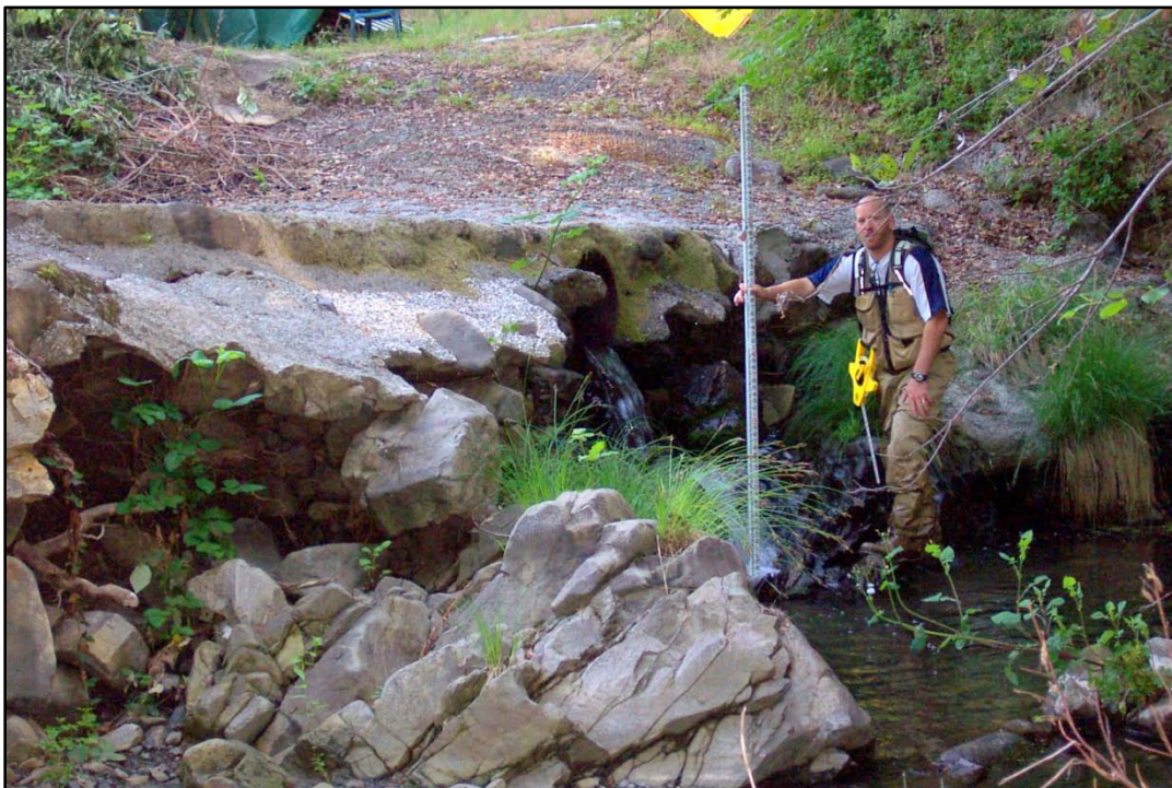
Figure 3. View of downstream face of Pickle Canyon Creek concrete ford under low flow.
