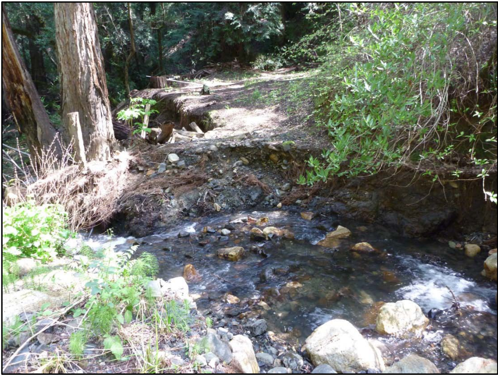
Figure 11. Looking across the earthen ford toward the right bank. Downcutting of channel through trapped gravels.
