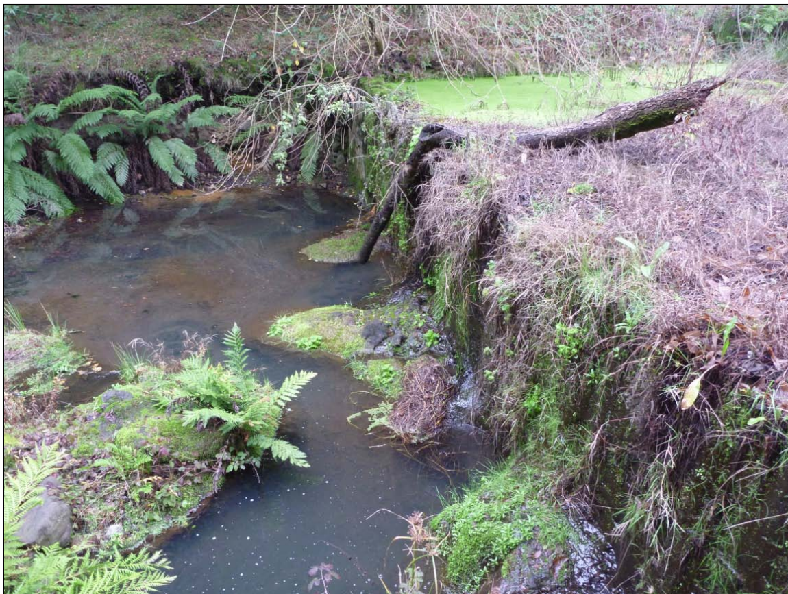
Figure 2. View of the dam from the left bank under low flow conditions.
