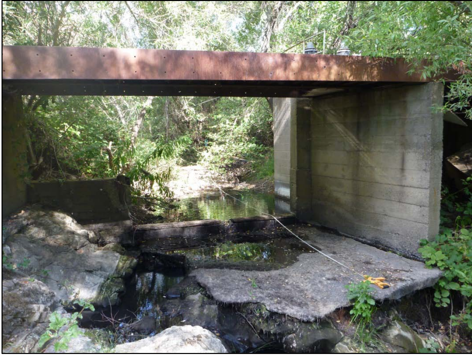
Figure 3. Looking upstream at the pumping station under summer low-flow conditions. Weir, apron, and bridge are shown.
