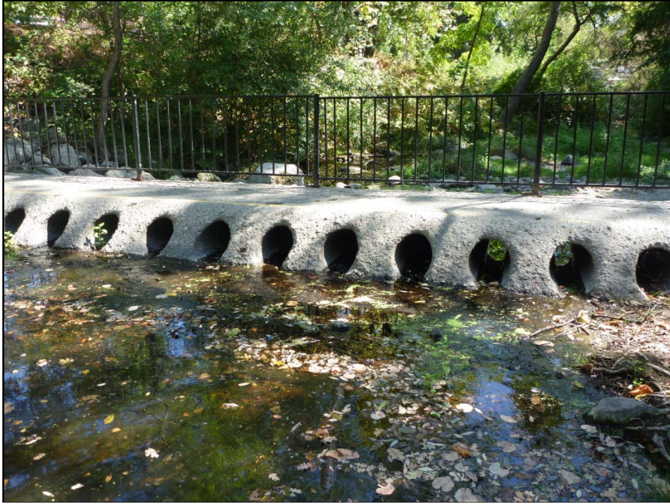
Figure 4. Closer look at upstream side of foot path under near zero-flow conditions.
