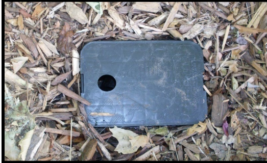
Small valve box
