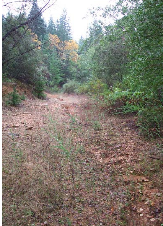
Figure 4. View of a gully down the roadbed at site #22.
