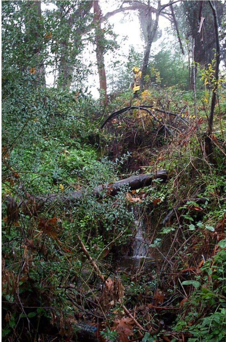
Figure 6. Gully down hillslope below the pond overflow culvert at site #6.
