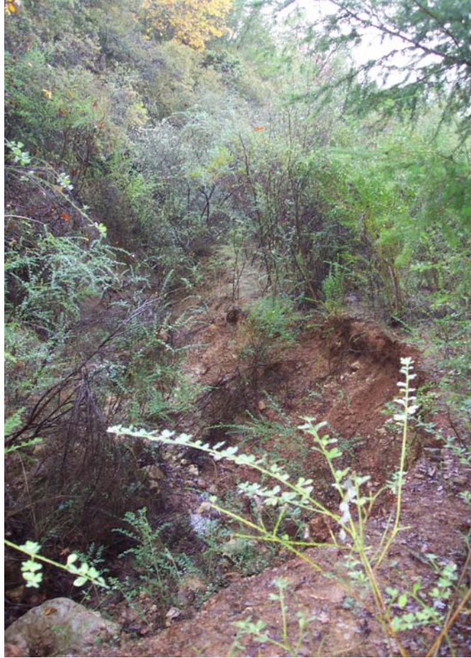
Figure 7. Gully from diverted stream at site #30. Proposed treatment is to excavate the fill at the stream crossing.
