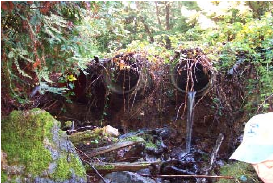
Figure 5. Two concrete 36" culverts and 1 steel 36" culverts and sandbag crossing at site #11 on Wing Canyon. Decommission of crossing fill is proposed.
